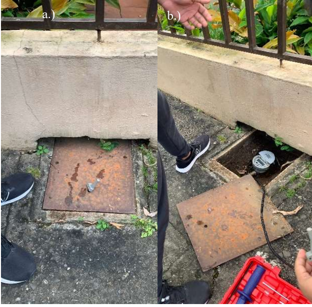
Fig. 4 Installation site of water meter 32862704. (a) Normal aspect of meter casing with protruding antenna from metal casing. (b) Meter casing opened for service.
