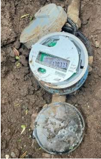
Fig. 2 Damaged water meter (32862702) installed at a home in Betania
