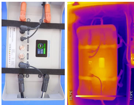
Fig. 9 External temperature behavior for the prismatic LiFePO 4 (16 cells in series and one parallel cells).
